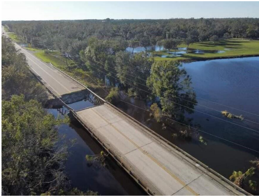
Figure 35: A portion of the Highway 64 bridge near Pioneer Park in Hardee County collapsed due to Hurricane Ian
