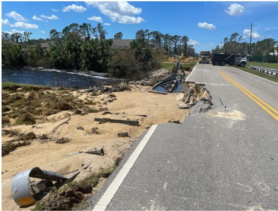
Figure 17: Roadway damage and partial washout near the Myakka River in North Port, Florida 89
